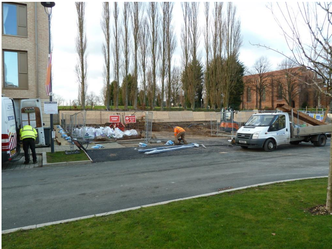
Preliminary works at the site of Cocoa House. The chocolate orange sculpture has been moved to Bayldon Square, January 2019. St. Chad's Church and the disputed poplar trees are in the background.
