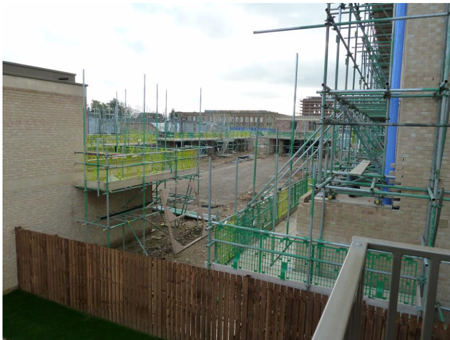
A sea of scaffolding. View from the [then] show house on Clock Tower Way towards the Terry's HQ Building. November 2015.
