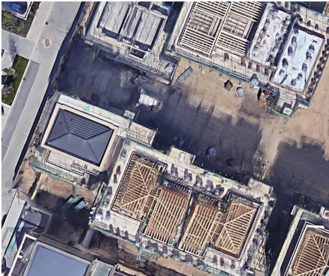
The air photo above (Google Earth) shows the northern end of Robert Street under construction. The central group of four townhouses at the bottom have been completed to roof level.
