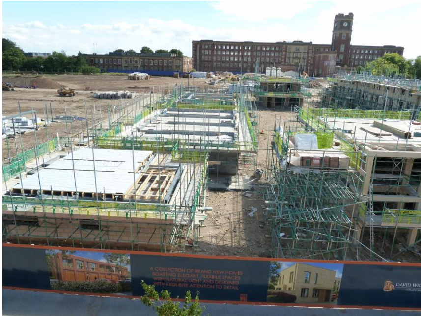
This photo shows progress on the David Wilson Homes site in early August 2015. It was taken from a balcony on Neapolitan House. The large house in the foreground to the left of the picture is No. 2 Robert Street.
