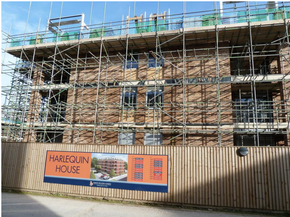
Harlequin House at third floor stage, showing the progress of sales, February 2019.
