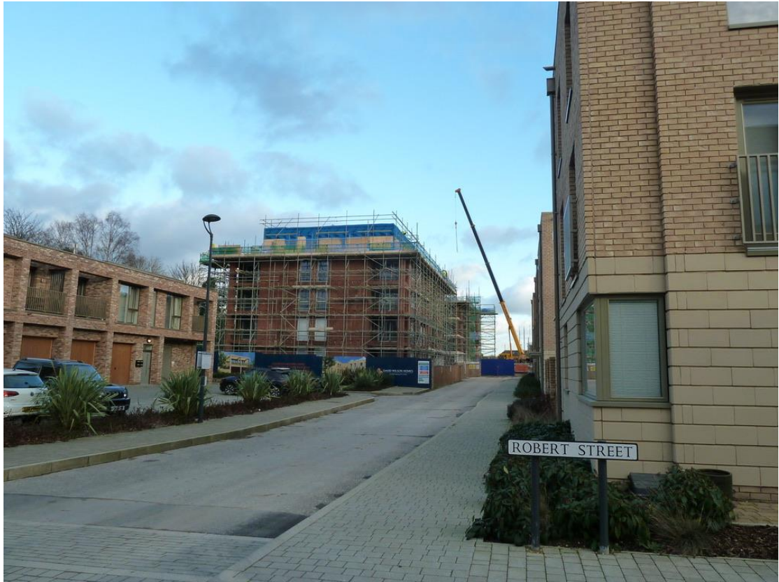
Joseph Terry Grove looking east from Robert Street. Devon and Carousel Houses are nearing completion, January 2019.
