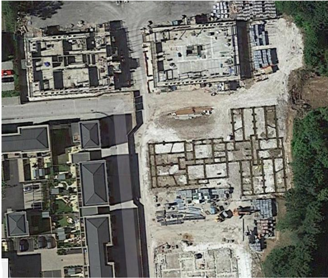
Work in progress on the site around October 2018 (Google Earth). Work on Blocks C (Devon House top left) and D (Carousel House top right) is well under way. Block E (Medallion House centre right) is at foundation stage, while Block F (Harlequin House bottom right) has barely started.
