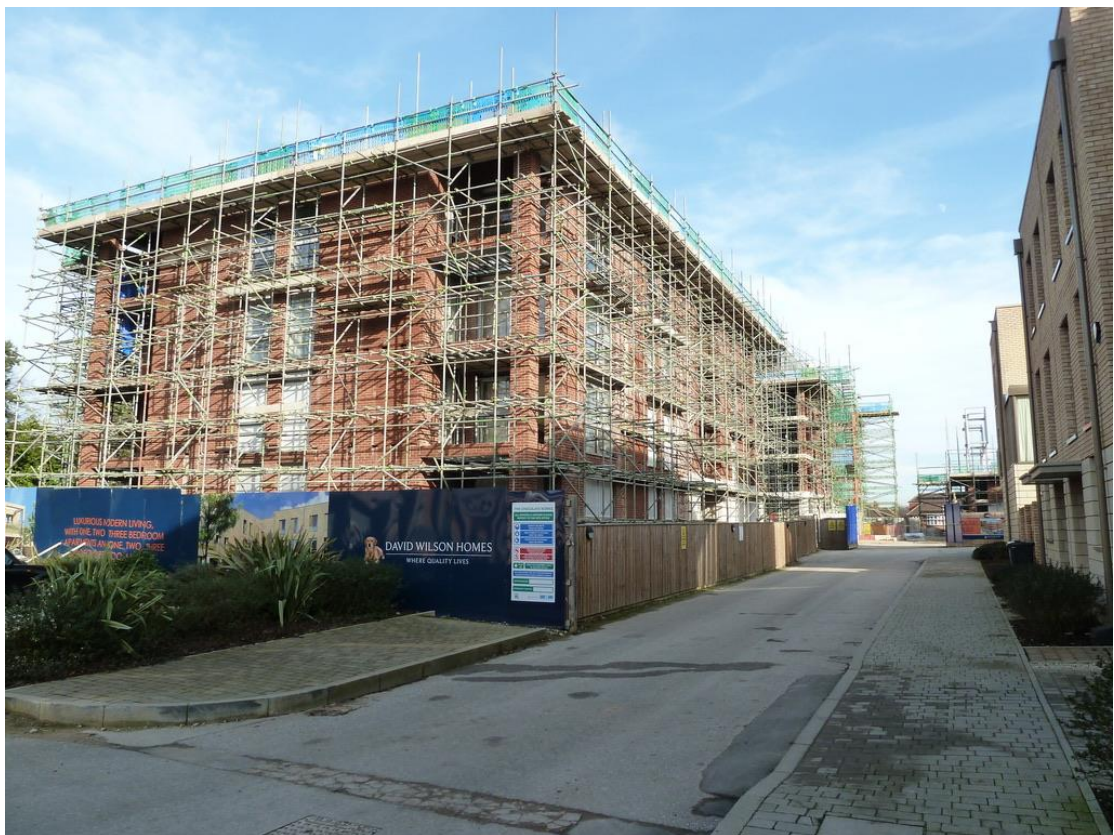
Looking south along Joseph Terry Grove. Medallion House in the foreground. February 2019.
