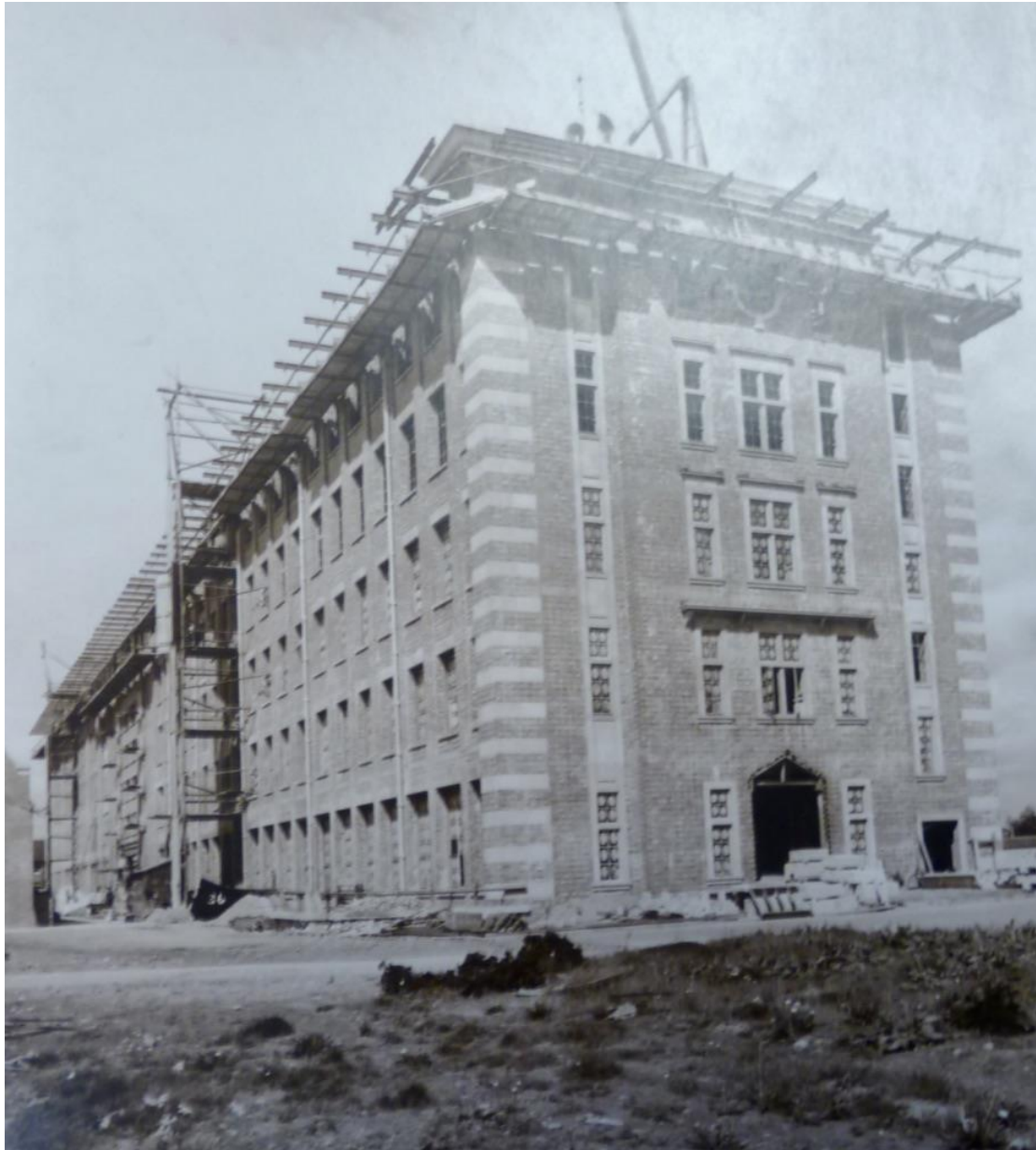
The main factory under construction. Probably around 1926. Courtesy of the Borthwick Archive.
